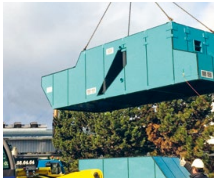
The new boiler installation in Souvans
